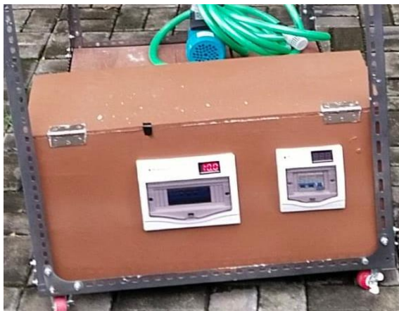
Gambar 4.3 box panel control
